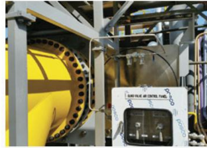
Coke Oven Gas(AOV automation)
