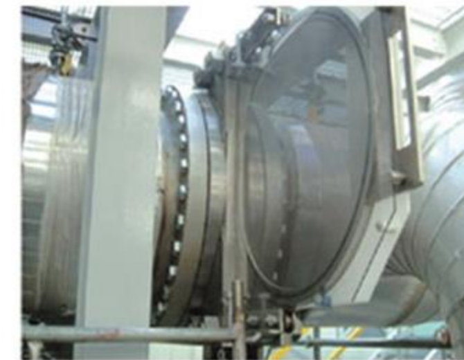
Heat Exchanger-Bypass Line
